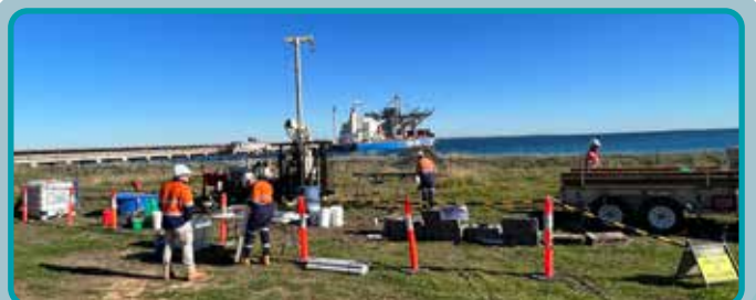
Geotechnical investigations in Kwinana Industrial Area. Image supplied by Fremantle Ports Authority.
